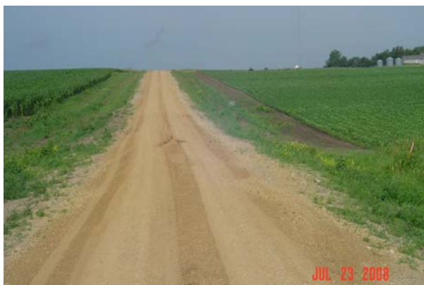
Figure 12: Duel County Example of Road Deterioration Under Development Traffic (from top: original access road; failed access road; failed alternate route, repaired access road)
